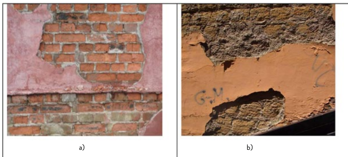
Figure 1 - Destruction masonry under plaster layer: a) Moscow, Russia; b) Naples, Italy.
