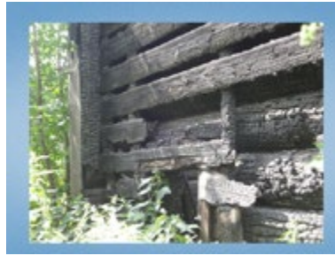
Figure 15 - Log house with planking of wooden boards after the fire. It is clearly seen in the photograph that there is an air gap between the logs and the wooden boards along the bars
